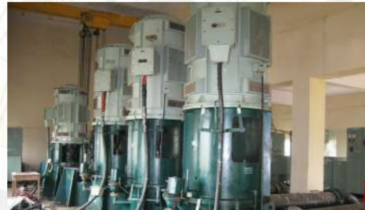
Lift Irrigation System Pumpstation
